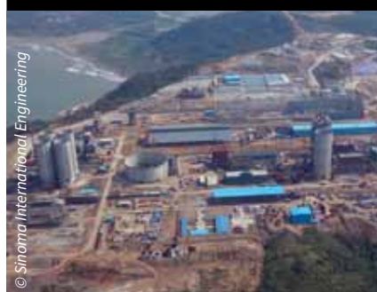
As Western cement producers exit the region, plant construction is increasingly undertaken by Chinese contractors such as Sinoma International Engineering Co Ltd
